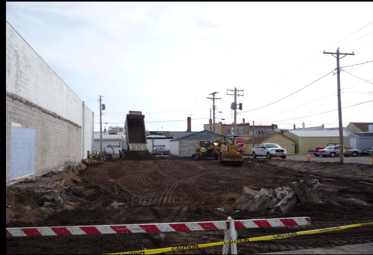
Old Laundromat building is now history. Crews are working to complete a parking lot for AMPI.
